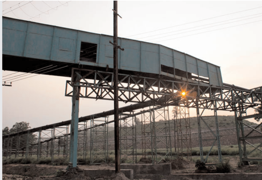
Pipes like these carry treated, mildly radioactive slurry from Uranium Corp. of India's mining operations to a system of uranium tailing ponds covering 193 acres. The company says it posts proper signs warning locals not to trespass.
